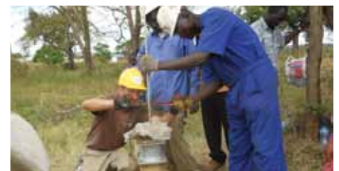
Lifewater field trainer Doug Headrick works on an India Mark II pump with technicians in Uganda.
