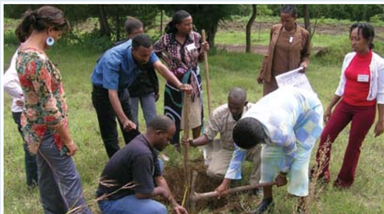
Below: Ethiopian sanitation promoters work in teams as they apply their new knowledge in latrine construction.
